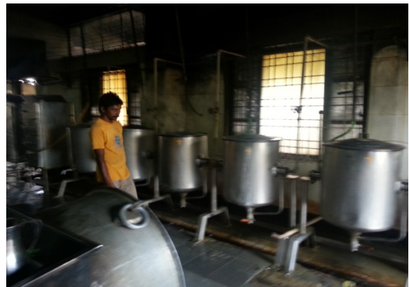
Cooking System at BPS
