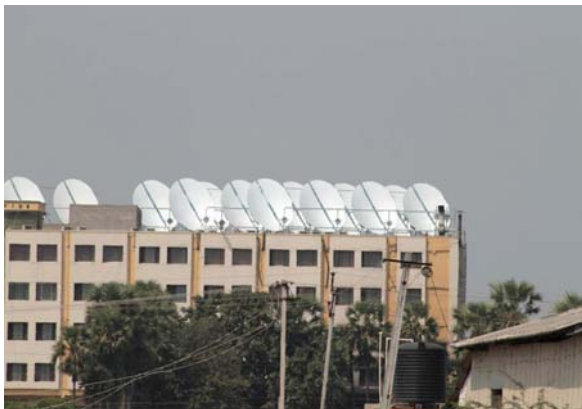
CST dishes on rooftop at Bhashyam School
