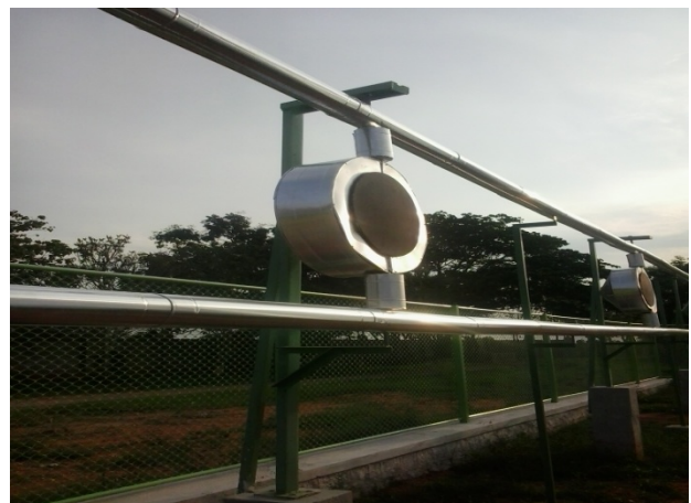
Heat receiver water piping
